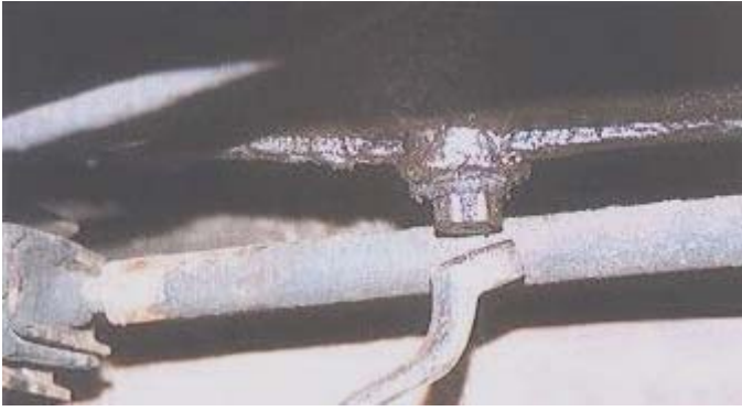
5) Undoing the gearbox drain plug, located just in front of the gearbox mounting cross-member.
